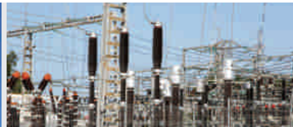
Electricity Power Station
